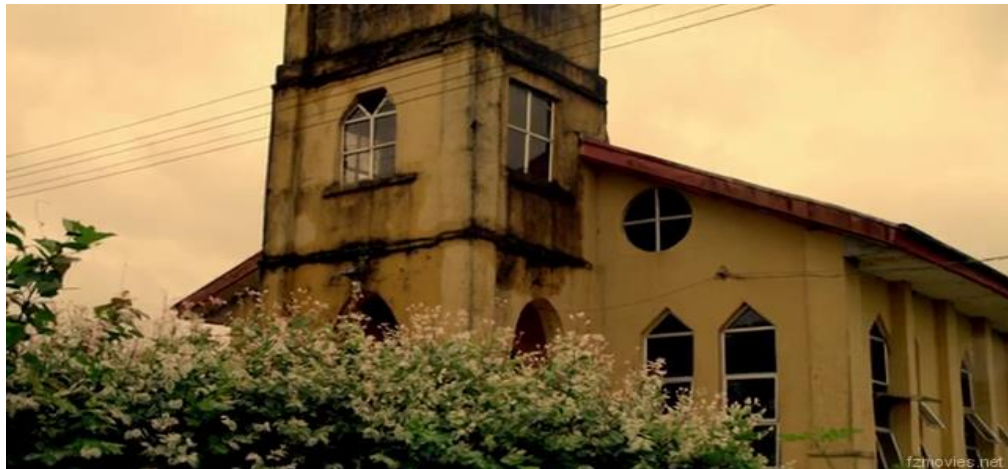
Snapshot 13 is a dilapidated and crumbling church building in the host community
