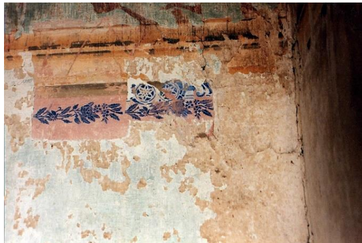
Figure 8. Ornament B, appearance of the walls before the intervention; note the ornamental borders with decorative motifs, found under several layers of thermoplastic paint. Photograph by the author (1999).
